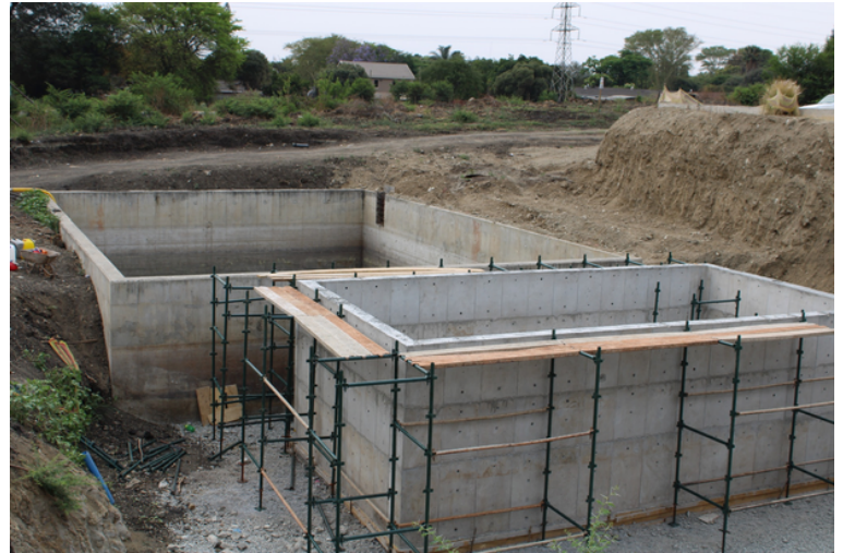
Some of the storage tanks which have been built and are due for mechanical and electrical works to be completed the end of the third quarter of the 2022/23 financial year.
