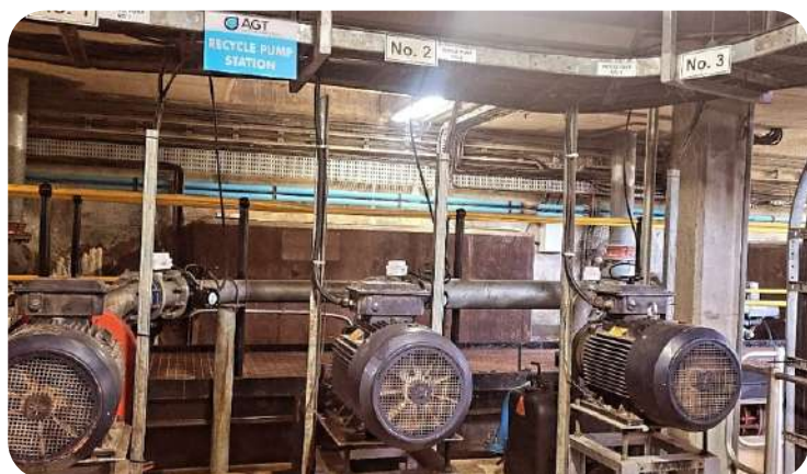
Pumps inside the Mmabatho WTW
